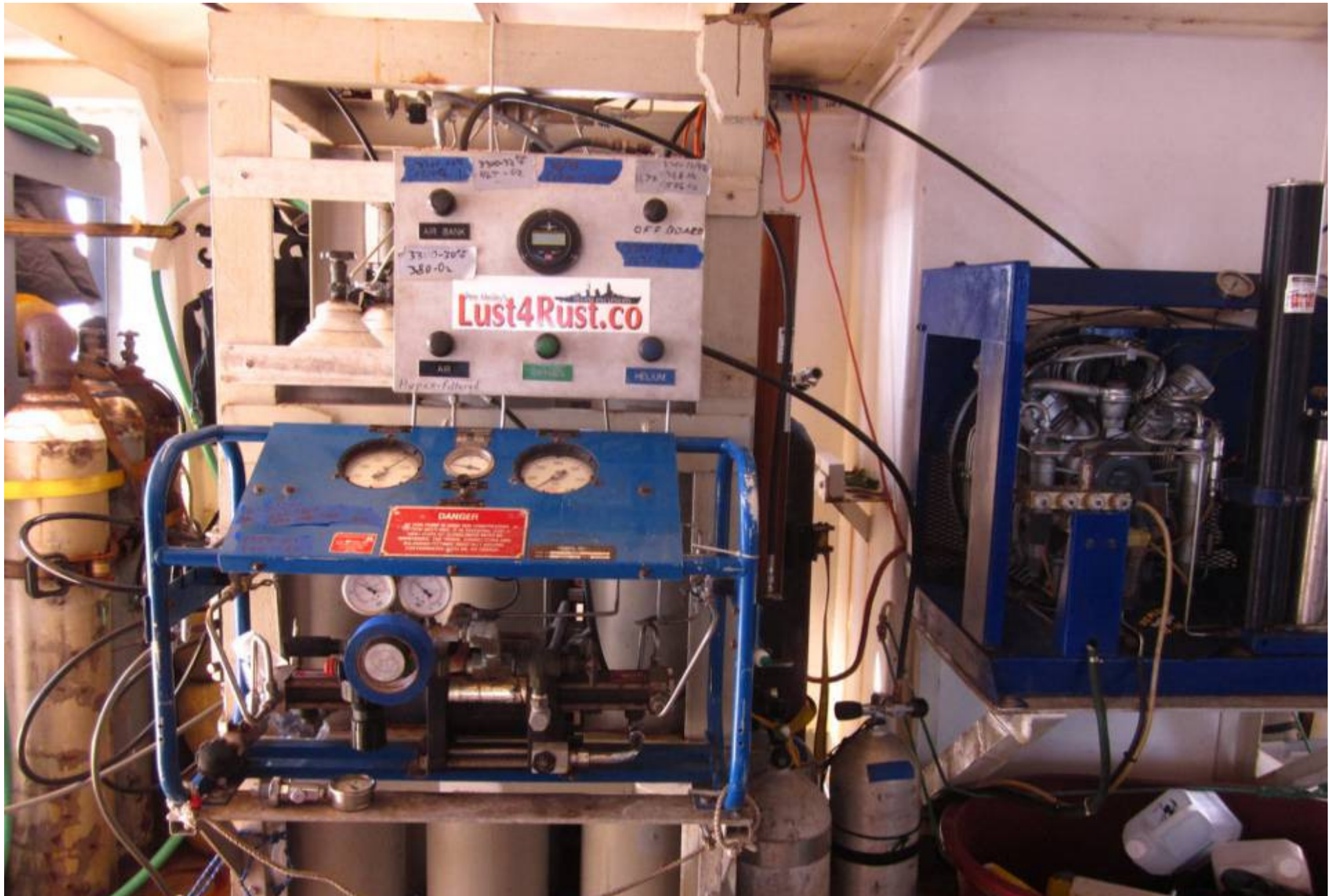
Onboard Tri-mix Tank Fills & Rebreather Support
