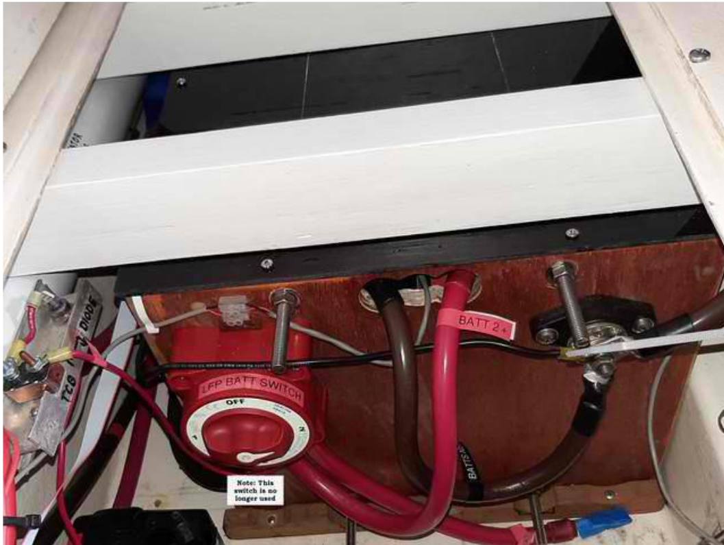
Front of our battery box, cover on and secured. Red cable is positive and brown negative. Small gray wire is solar MPPT sense.
