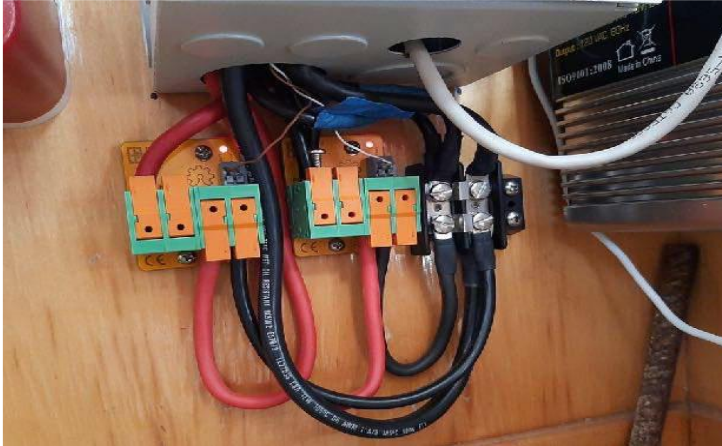
Two ElectroDacus DSSR20's provide HVD for solar panels
