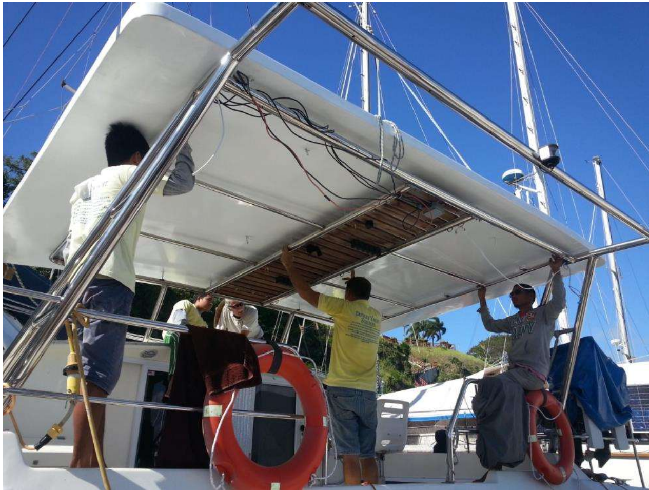
Water Catchment & 800 Watts of Solar
