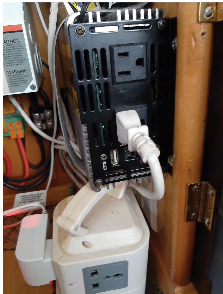
A Micro Solar 600-watt PSW inverter.
